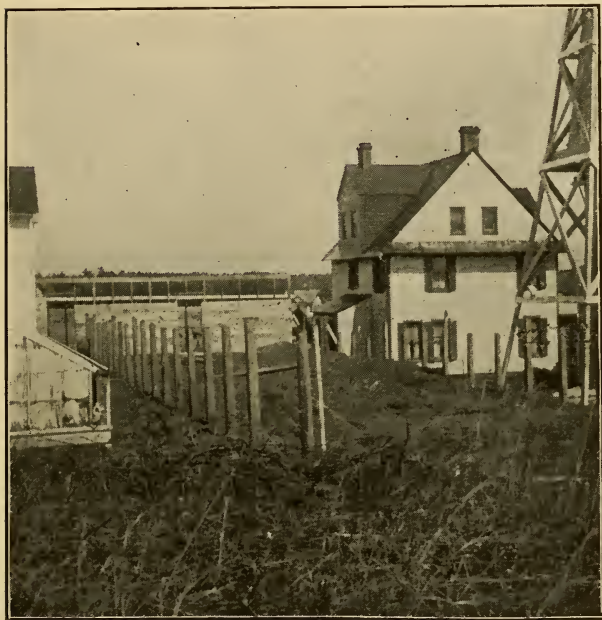
25.—House twenty-four feet wide; posts set and shed at north end built first
